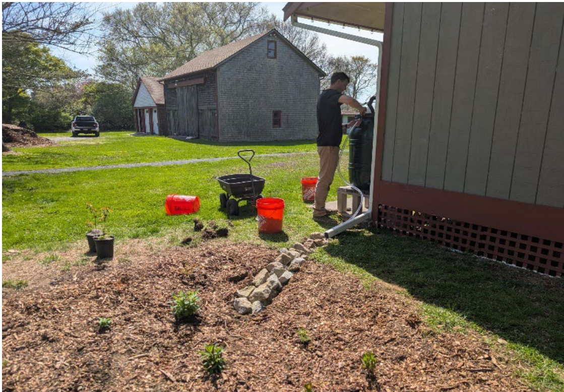
Prepping the inlet from the gutter and rain barrel into the rain garden.
